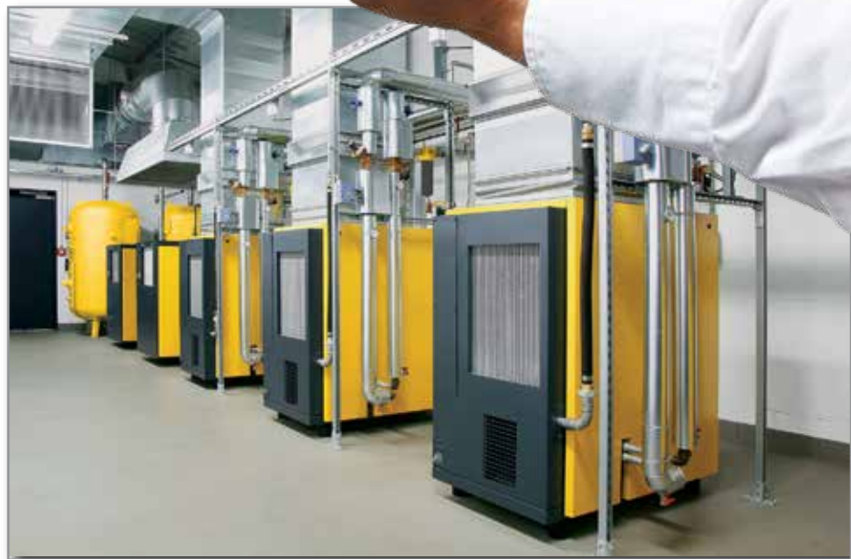
Air-cooled, fluid-injected screw compressors with internal heat exchangers and controls to tap into the thermal energy of the cooling fluid. The additional ducting removes the hot air that was not rejected by the hot water recovery system.
